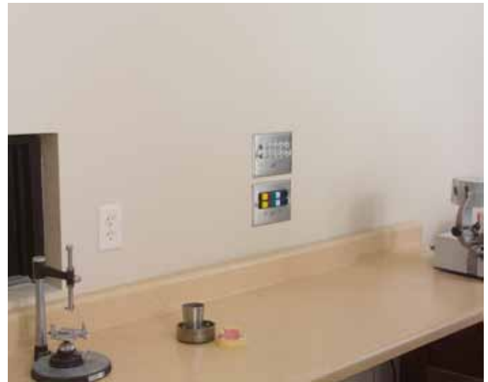
Fig #15 CRL169-2 Channel Hygiene Status Display and CRL 152-2 Two Channel Lighting Pushbutton Panel
