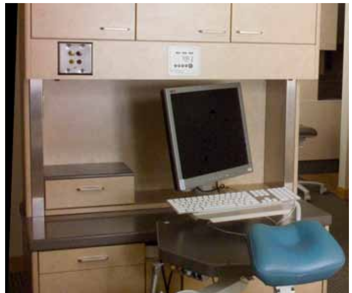
Fig #14 RSS 632 Two Light & Toggle Switch Panel on unit in Hygiene Operator CRL 130 Aluminum Button Bar is on tray table and CRL 160 Light Panel is on side wall
