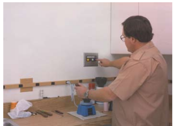
CRL 252 Lighting Pushbutton Panel
