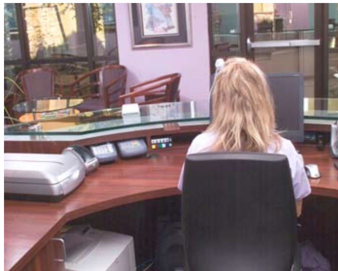
CRL 232 Lighting Pushbutton Bar in Reception
