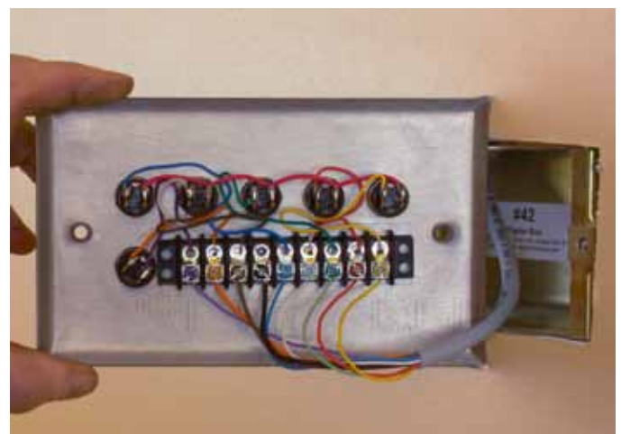
Wiring CRL 143 Button Panel on #42 Box
