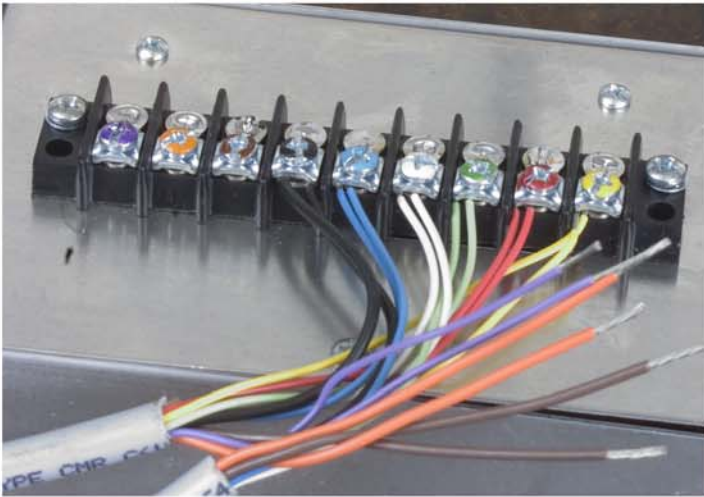
Connection of cable to terminals
